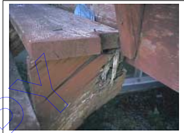
Rotted deck stairway stringers.
